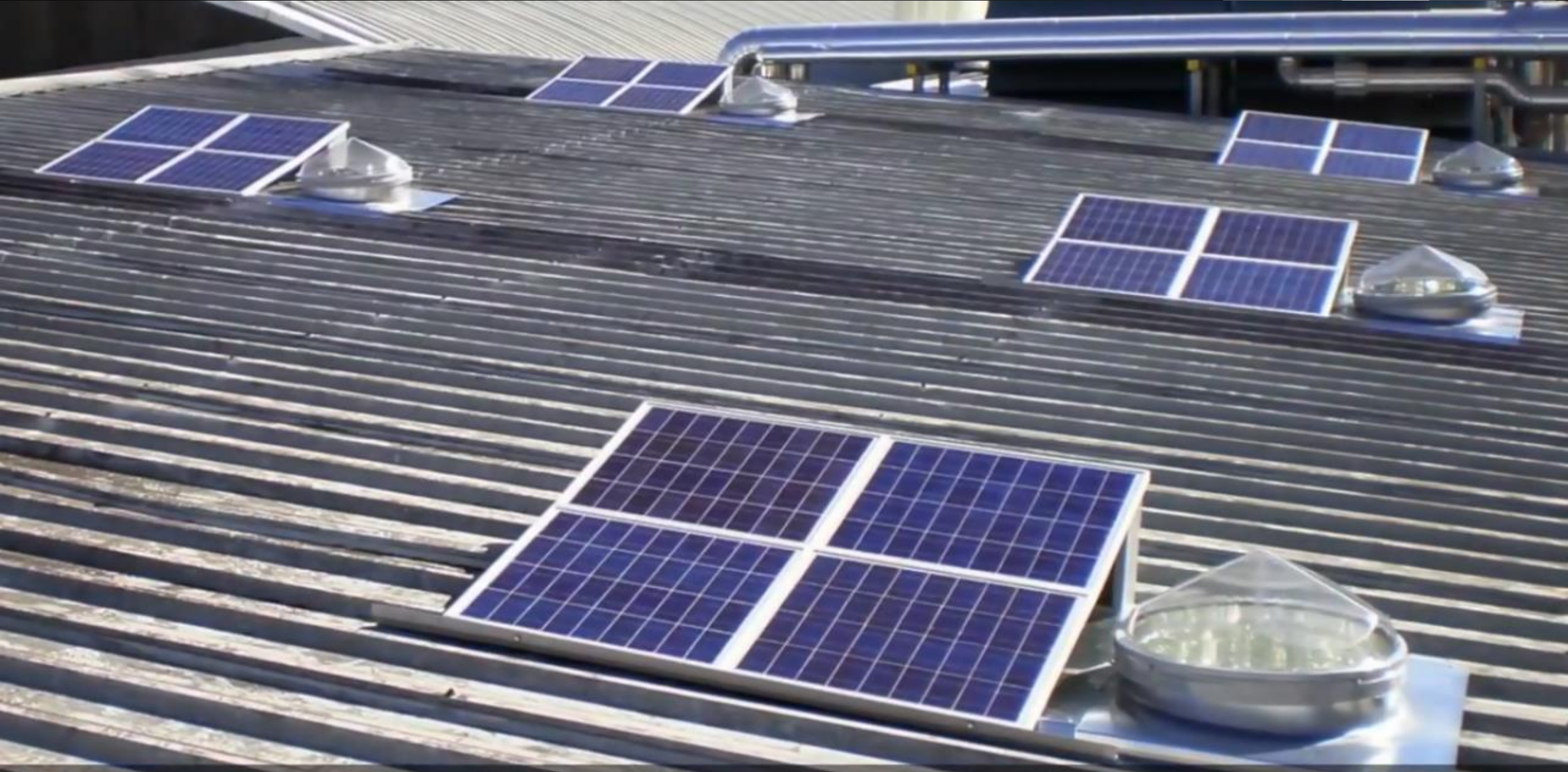
with the integration of a PV panel and a battery
